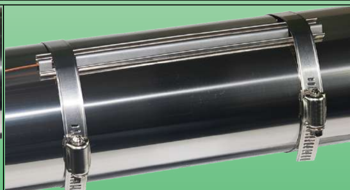
Example of the thermostat bulb model after installation
