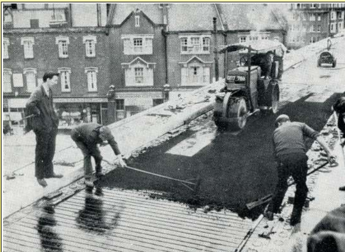
1969 Laying asphalt on the upper carriageway of a Hammerschmidt junction in London ( Electric heating of the roadways, by Robert Félix, 1971, Ultimheat Museum* )
